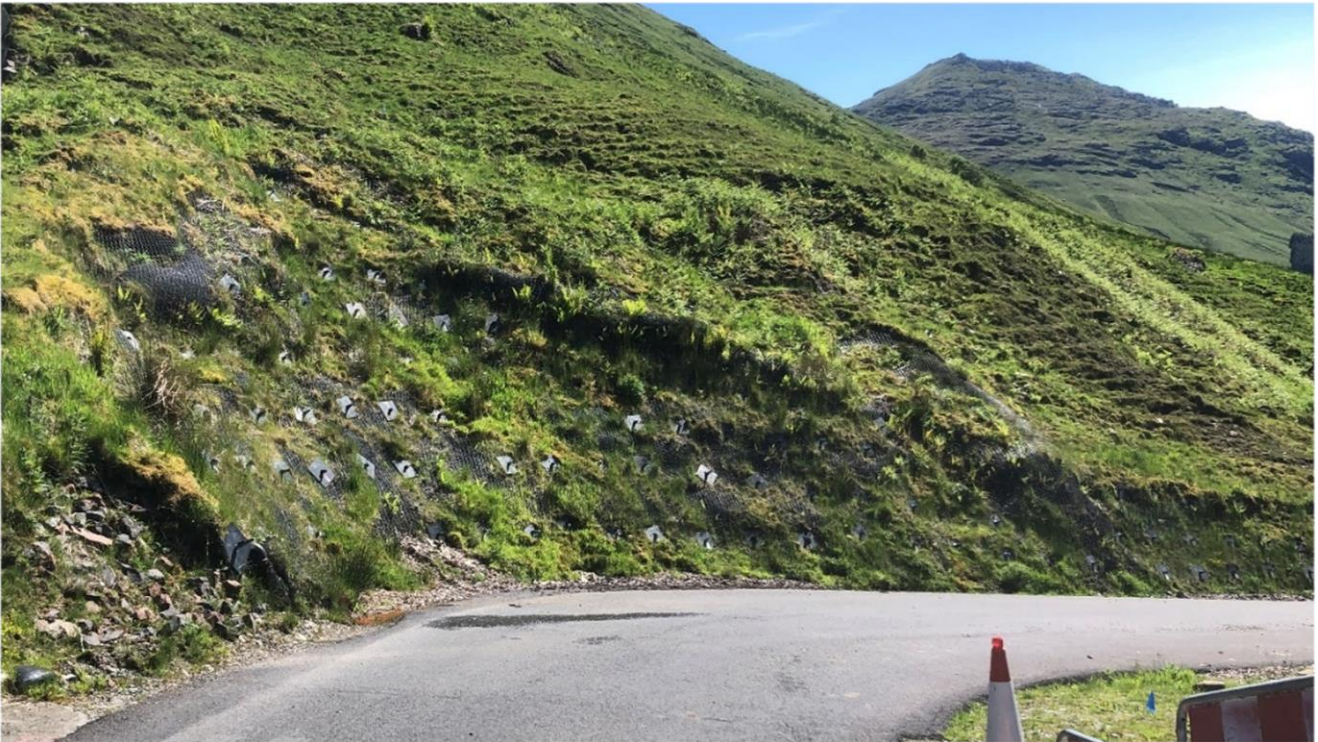
Figure 2-3 – Existing soil nailed slope above the OMR, looking east with The Cobbler in the background
