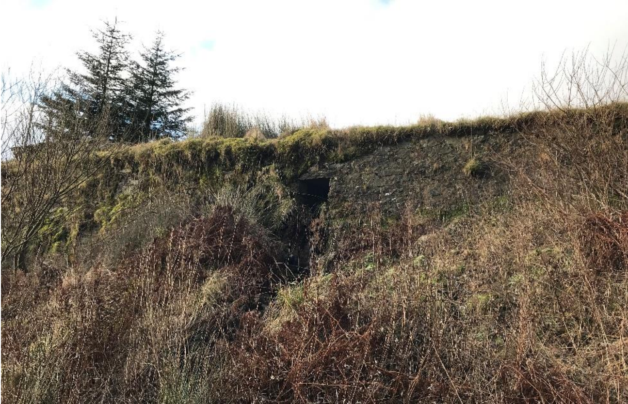
Figure 2-13 – OMR Retaining Wall 3, looking north towards the Rest and Be Thankful Viewpoint Car Park with vegetation in the foreground and trees in the background
