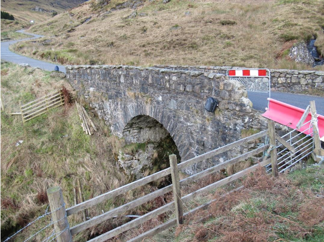
Figure 2-9 – OMR Bridge B, South-Western Elevation, looking north towards the Rest and Be Thankful Viewpoint car park
