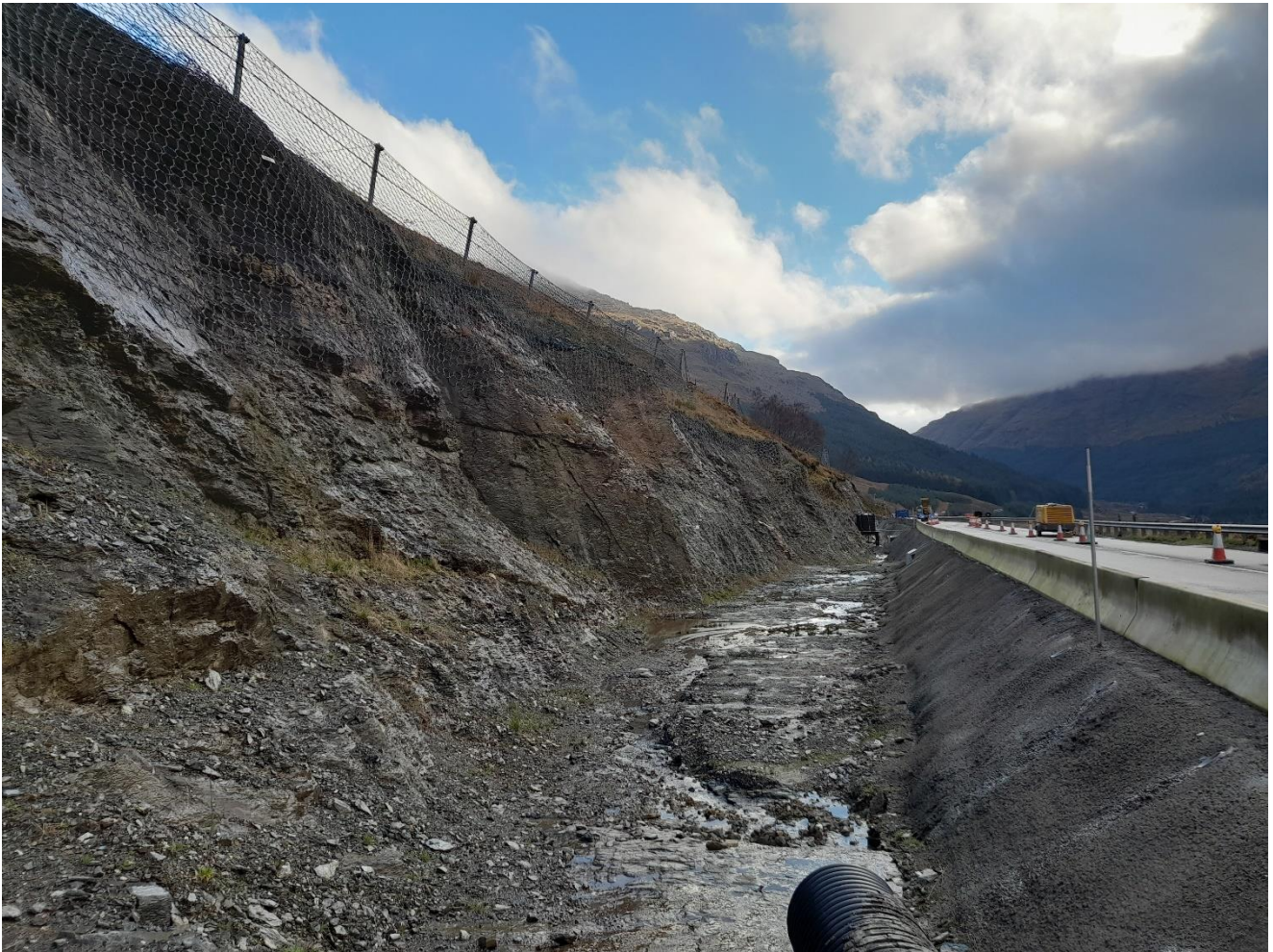
Figure 2-6 – Photograph of the extended catchpit adjacent to the A83, below the Beinn Luibhean hillside
