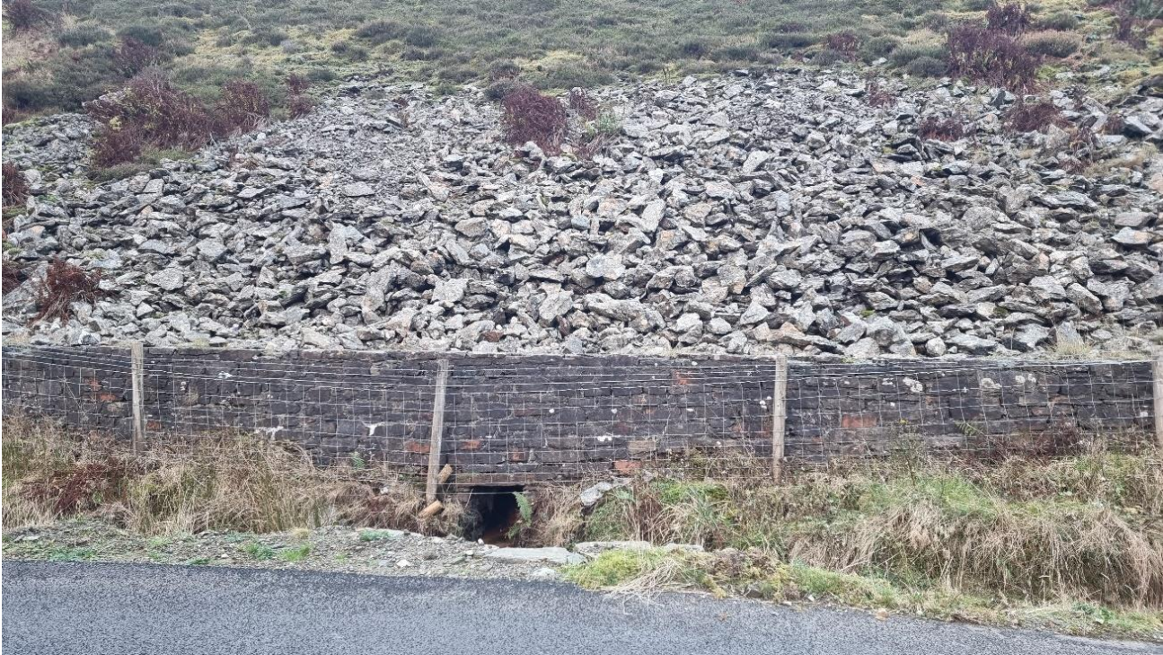
Figure 2-12 – OMR Retaining Wall 2, looking east with the lower slope of Beinn Luibhean above
