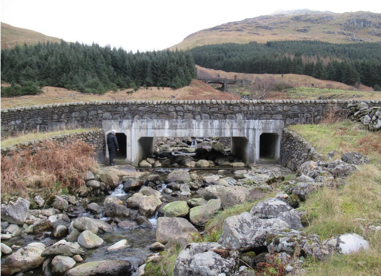
Figure 2-8 – OMR Bridge A, looking east up Croe Water towards the A83, with the A83, Cobbler Bridge and The Cobbler in the background
