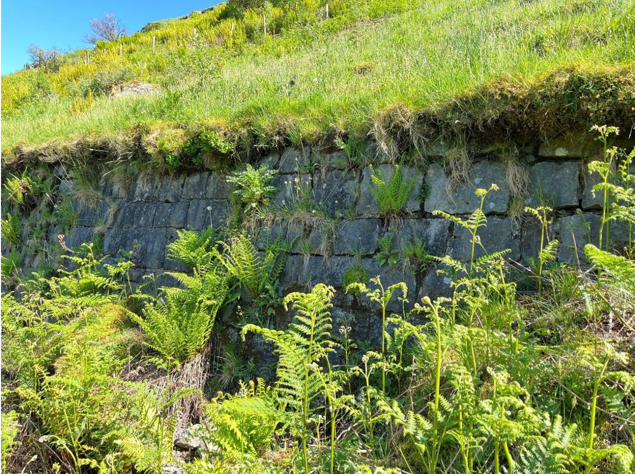
Figure 2-14 – OMR Retaining Wall 4, looking north towards the Rest and Be Thankful Viewpoint Car Park with vegetation in the foreground and grassed slopes in the background
