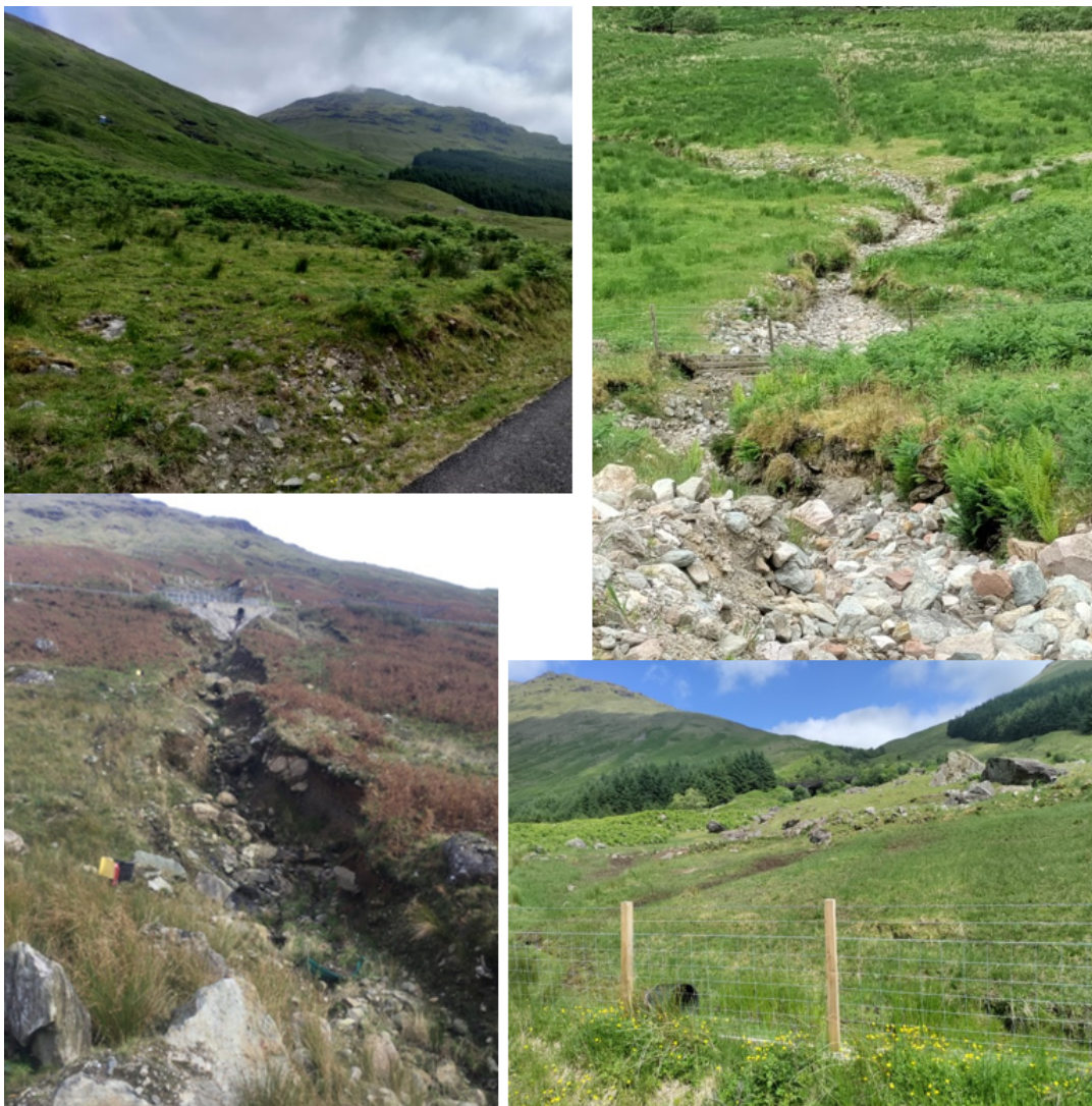
Plate 19. 7 - Selection of photos showing the slope downstream of the A83 which informed the baseline velocity selection for the assessment.
