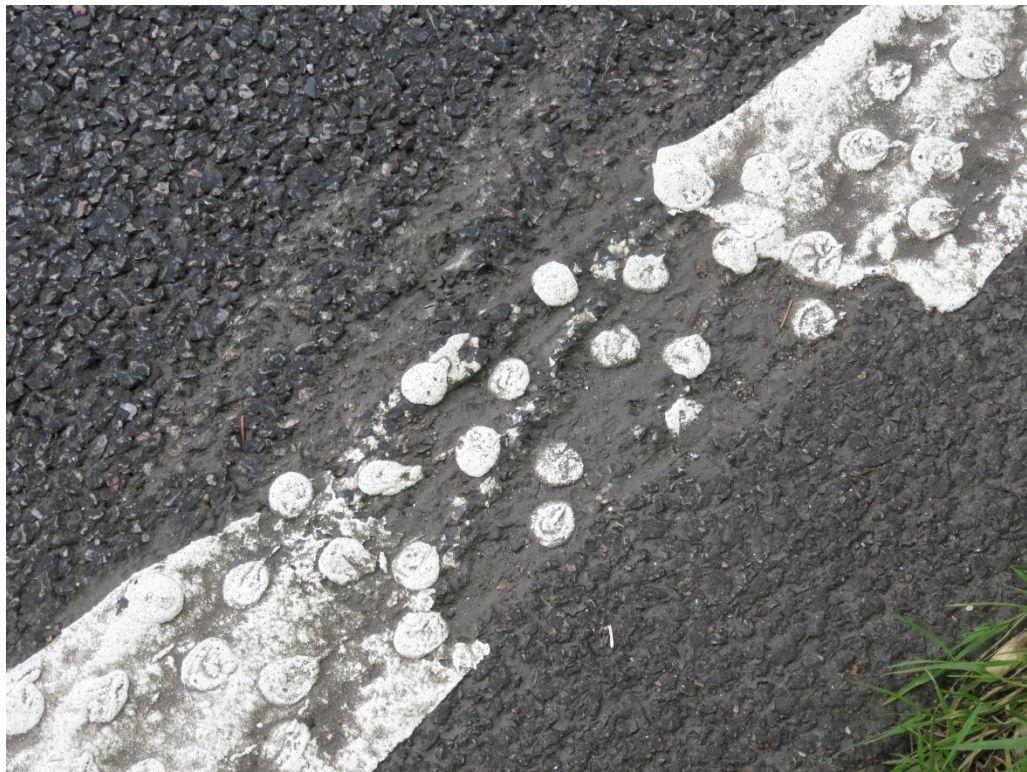
Figure 4-5 - Mechanical damage to surface course at IP28
