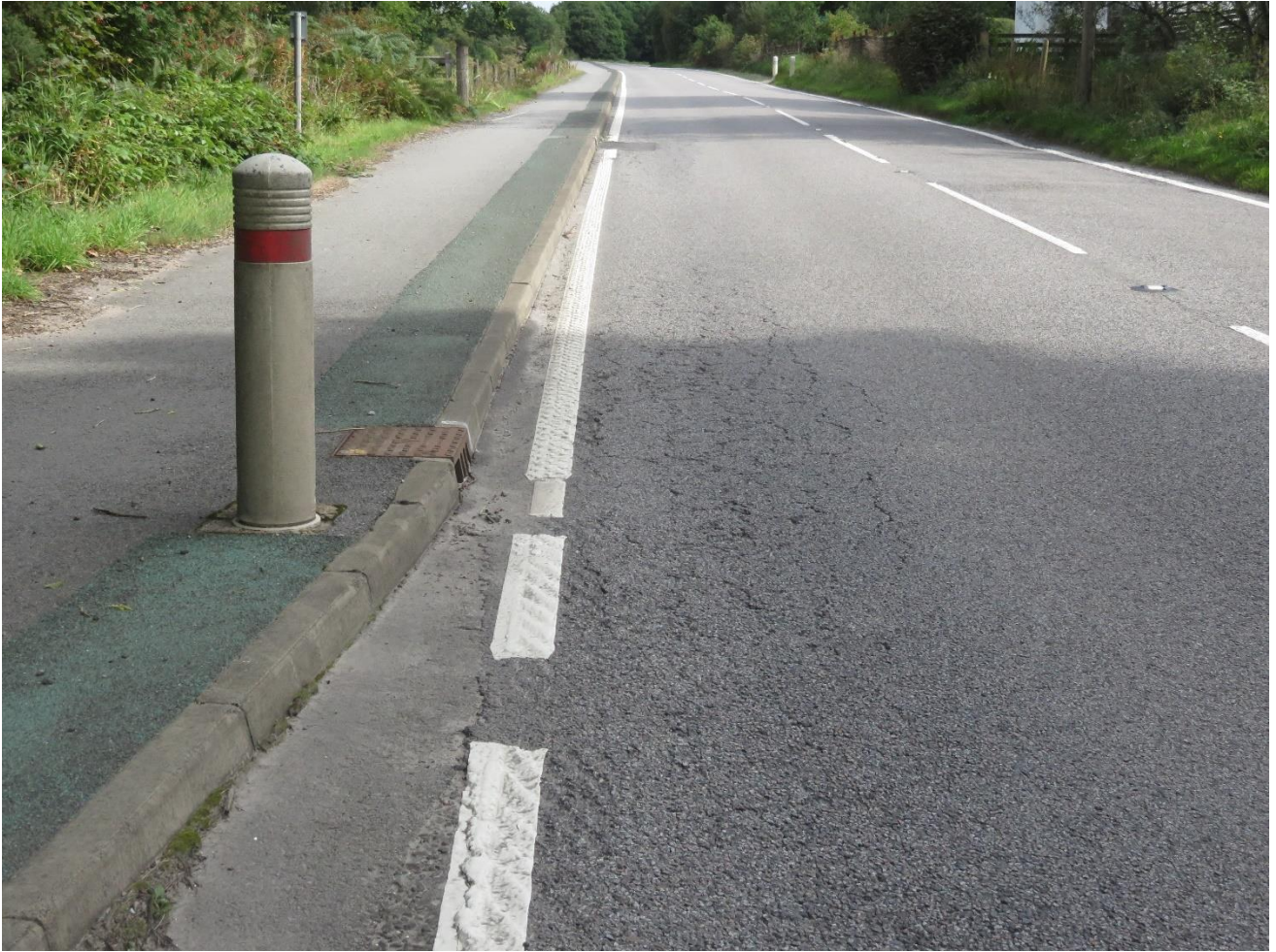
Figure 4-3 - Poor structural support at IP27
