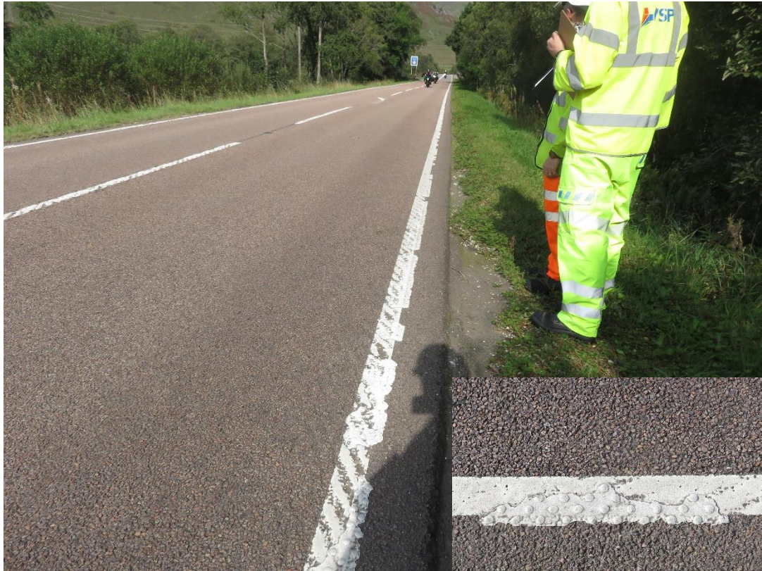
Figure 4-4 - Delamination of new marking material at IP25
