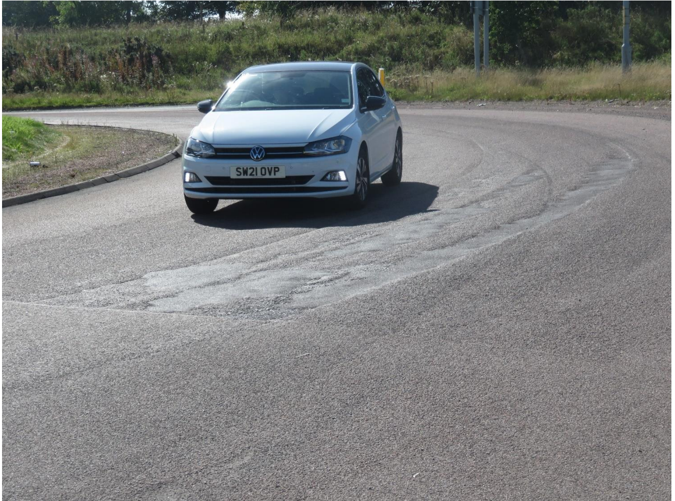
Figure 4-2 - Roundabout surfacing failure at IP40b
