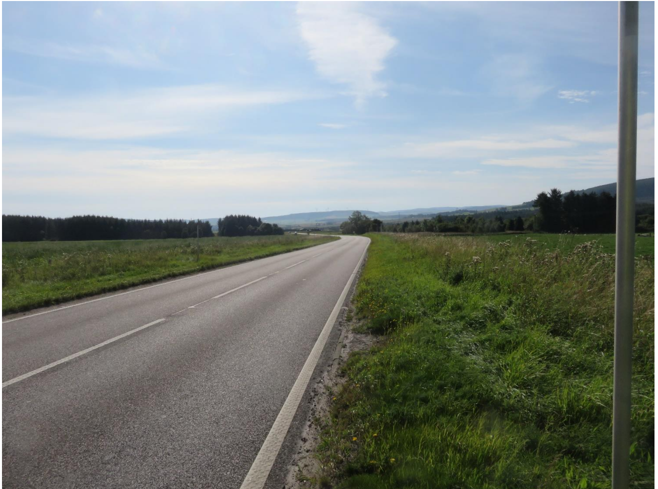
Figure 4-6 - IP37 assessed to be defect free after 5.3 years in service
