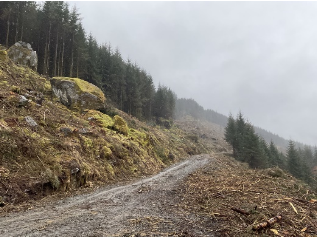
Photograph 25: Target Note ID - PM20, cavities present along the earth bank among the scattered rocks and piled earth.
