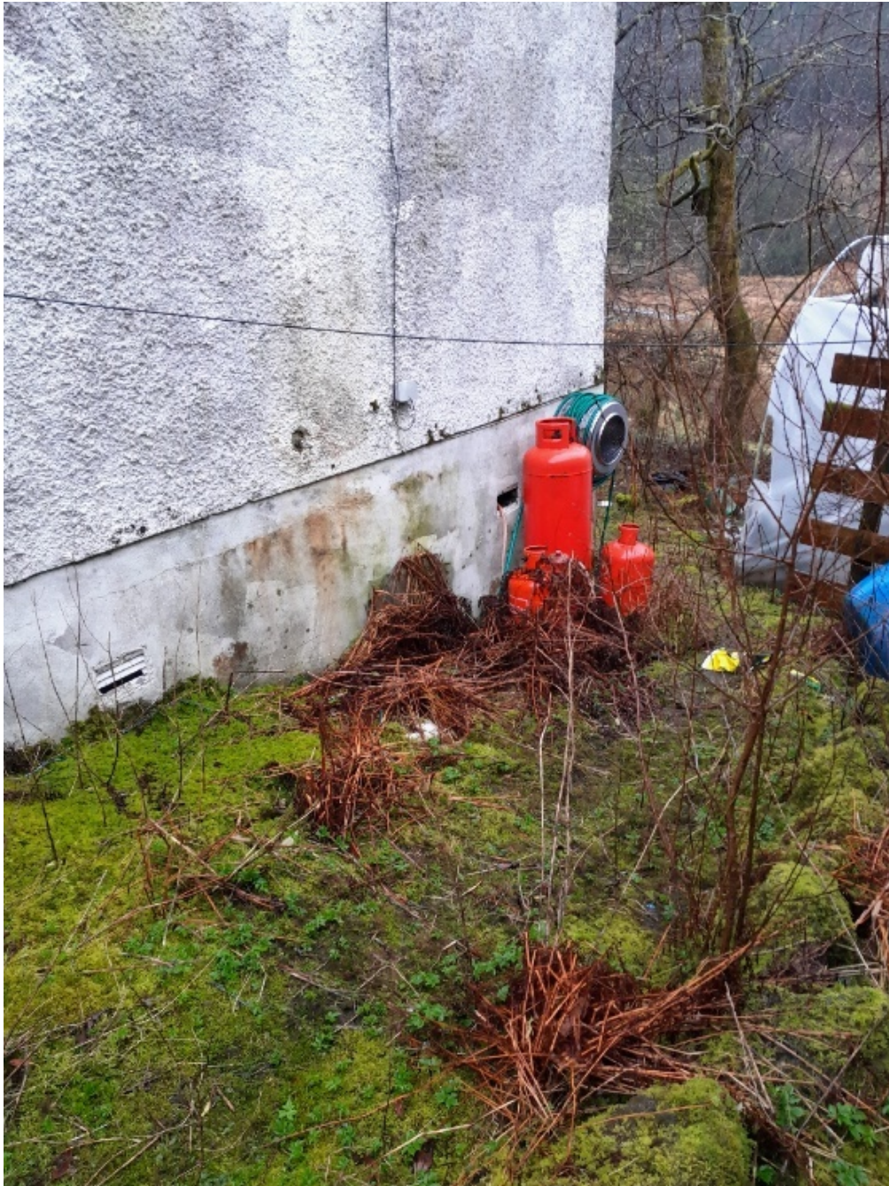
Photograph 14: Target Note ID – PM12, potential ingress point to abandoned cottage at ground level adjacent gas pipe exit.
