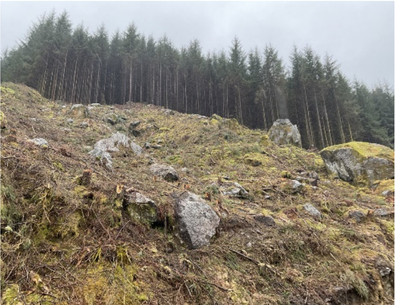
Photograph 24: Target Note ID - PM20, cavities present along the slope among the scattered rocks and piled earth.
