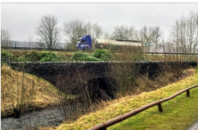
Photograph 15.24: Dowally Bridge (Asset 212) with traffic movement on the existing A9 visible in the background
