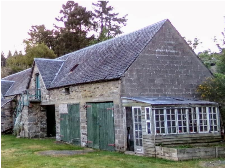
Photograph 15.14: Modern concrete block-work and lean-to, southern gable end of Guay Farmhouse Wing
